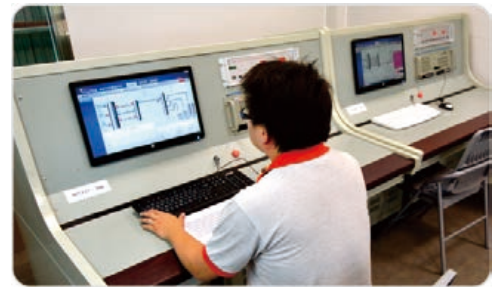
Control room & Graphical HMI
