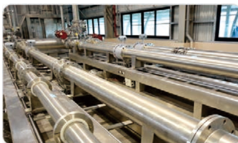
Piping system II (Maximum diameter is 300mm)
